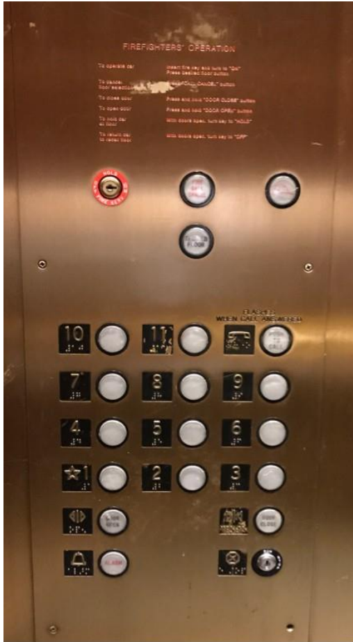
Figure 1. Elevator Control Panel in RISD Fleet Library
